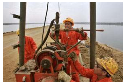
Construction workers bore a hole in the harbour bed at the site of the Hambantota port project, about 160km south of Colombo. Most of China's massive funding is meant for the port and a power plant. Gemunu Amarasinghe / AP Photo
